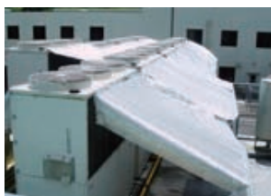
Shielded air-conditioner outdoor unit
