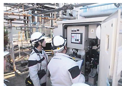
Power generator operation drill (BCP drill)
