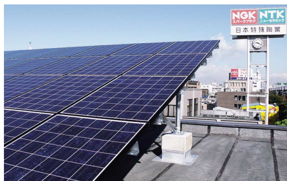
Photovoltaic generation panels
