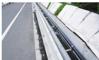
Miyanojo: Aboveground piping
