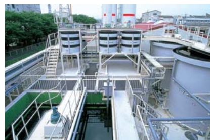
Effluent treatment plant at Komaki Factory
